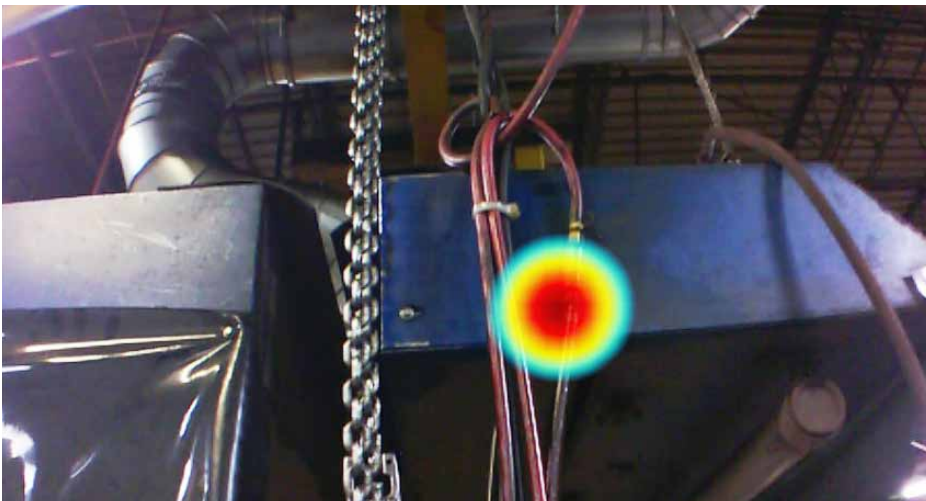
Image taken with the ii900 Industrial Acoustic Imager of an air leak in an industrial environment.
